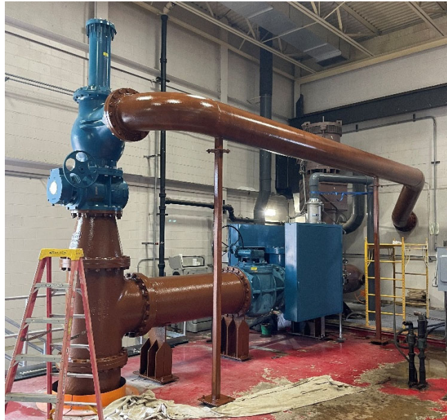
Photo A – New piping and valves at Building K
